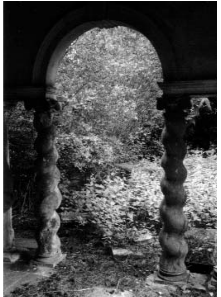
This close up reveals the decay setting in in the columns, probably imported from Italy. Still restorable though.
