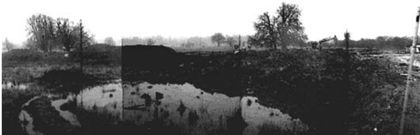
The parkland setting of the Grade II* listed park & garden at Hartwell House, February 1999
